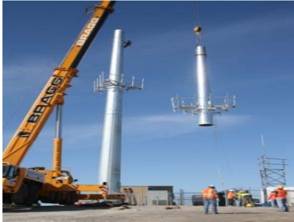
PATTERSON PASS MONOPOLE TOWER
